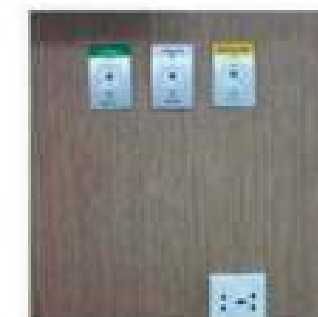
Built-in gas terminal and power outlet
